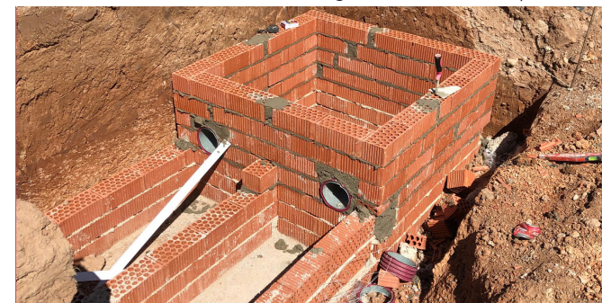
Water retention and monitoring chambers, Benicalap. Valencia
