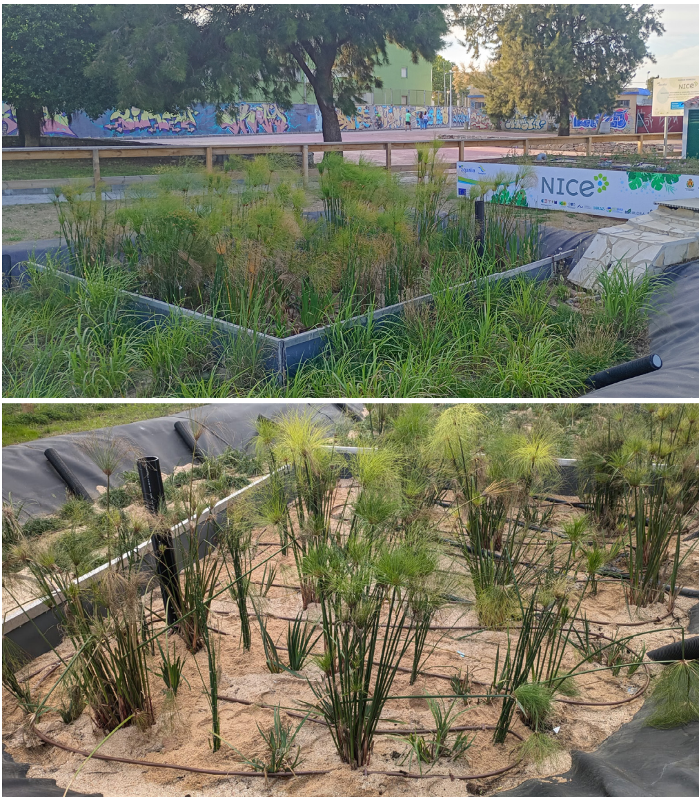
Figure 2.3.11 Installation photo of the wetland basin for grey water treatment.
